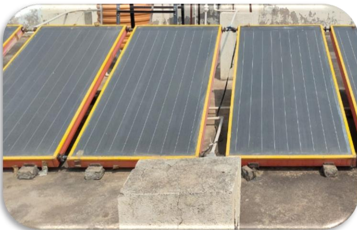
Solar water heating at rooftop of Hostel
