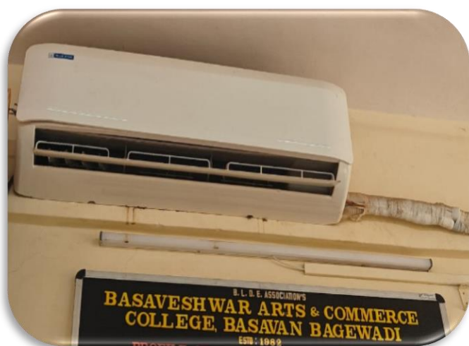
AC fitted in administrative section
