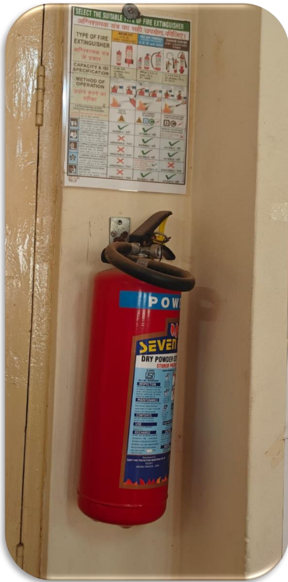
Fire Extinguisher at prominent places
